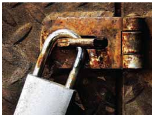
FITTINGS FROZEN BY RUST
